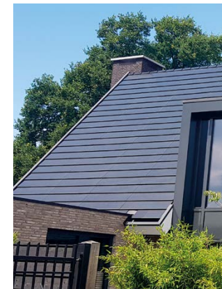
G 10 S PV-Solardach.
